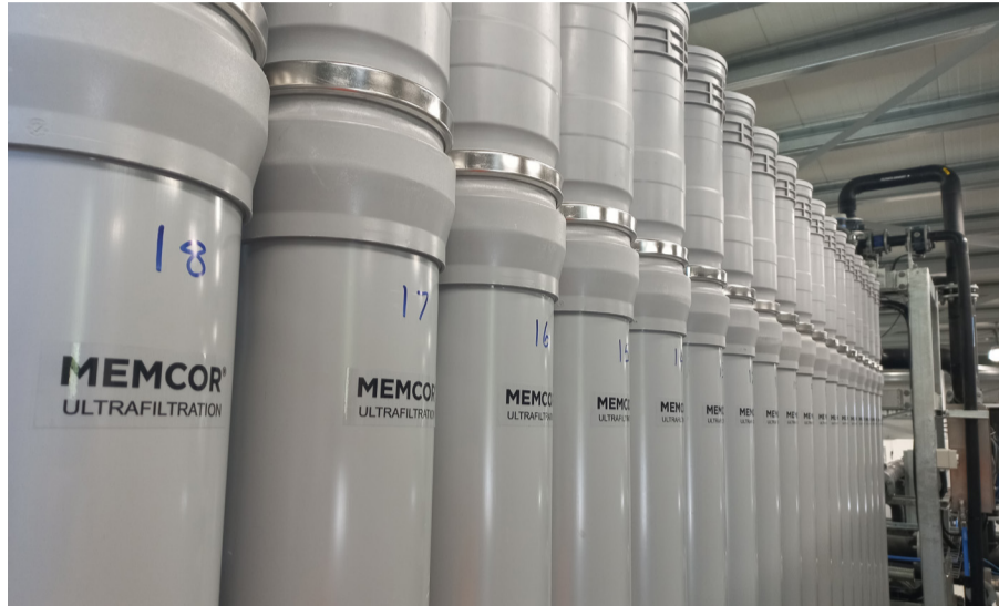
A row of membranes that now provide ultra filtration at the new $10m Methven Water Treatment Plant.
