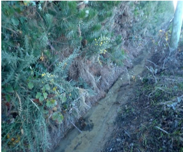
Figure c. Looking upstream at a dredged section of Willowby Water Race, flowing alongside Longbeach Road.
