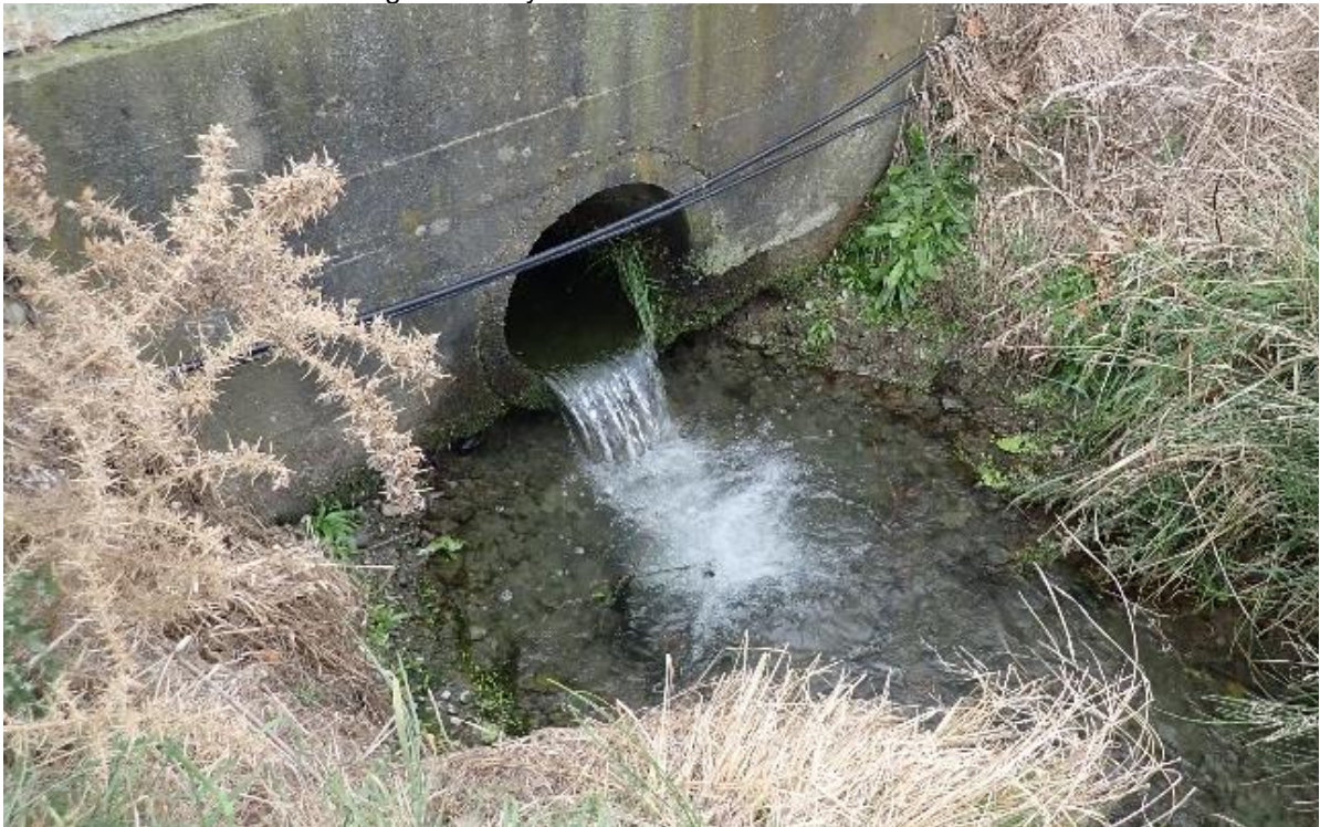
Figure k. Perched culvert across Boundary Road, at the downstream limit of ecological survey.
