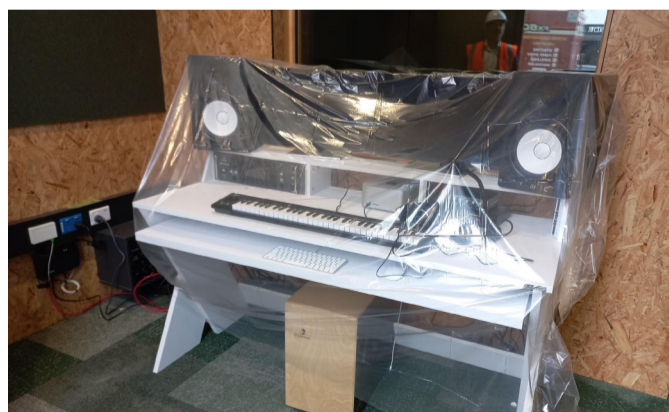
The library's new sound studio (left) and the new makerspace are nearing completion.
