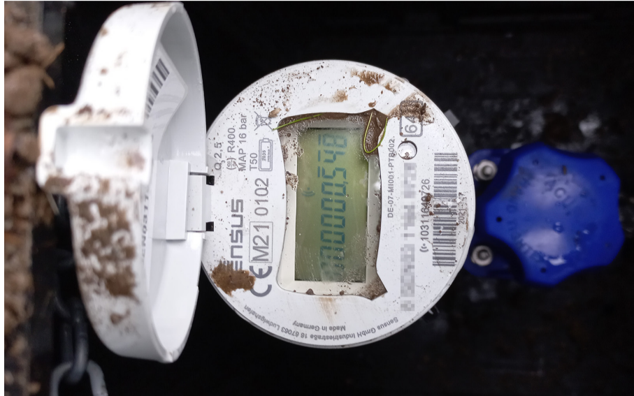
Readings from new smart water meters are highlighting potential water leaks.
