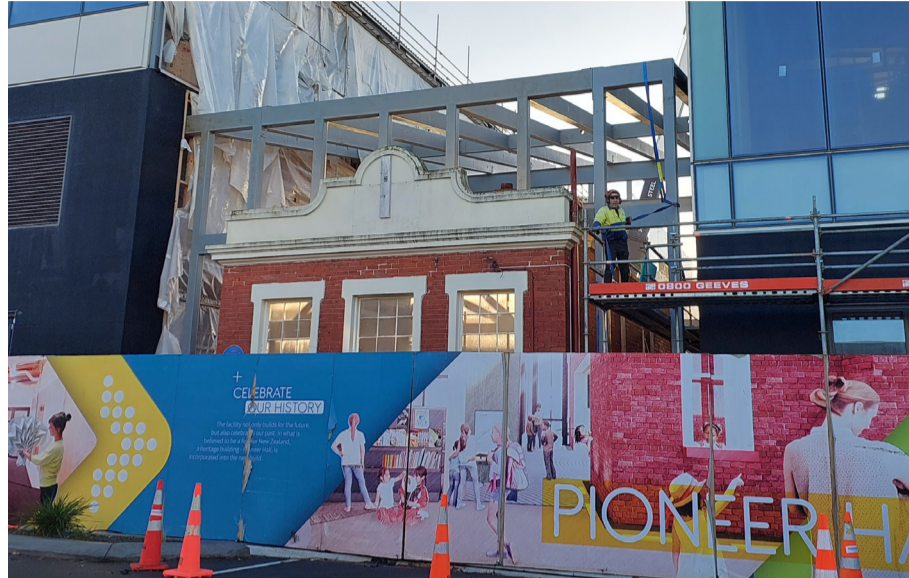
Pioneer Hall's historic facade becomes part of the new library and civic building.
