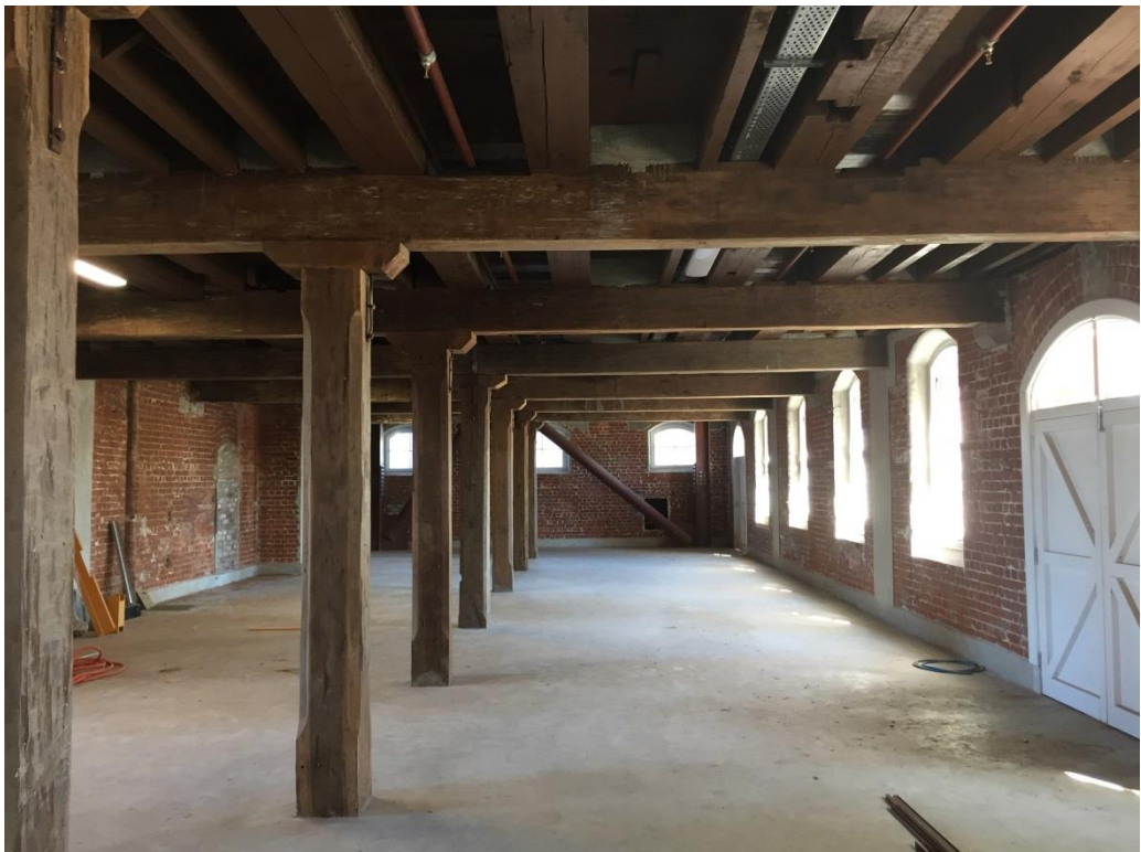
Figure 5. Woods Mill, Christchurch, 14 February 2019, Heritage New Zealand Pouhere Taonga photograph. Showing interior of four-storey mill building following structural upgrade (note steel cross beam).
