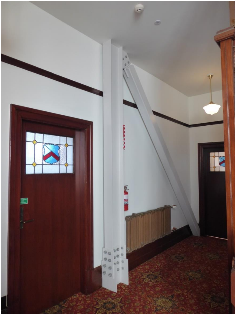
Figure 6. Midland Club (Former), Christchurch, 24 April 2018, Heritage New Zealand Pouhere Taonga photograph. Showing visible steel frame within interior spaces.
