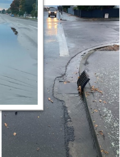
Team responding to Surface Flooding
