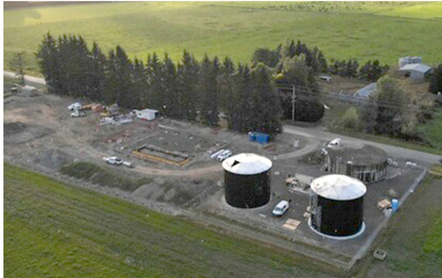
The two new reservoirs at the new Methven water treatment plant are ready for use, while a new building to house the new membrane treatment system is under construction.
