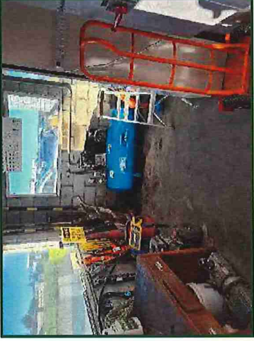
Photo 17 – Concrete control room with black staining
