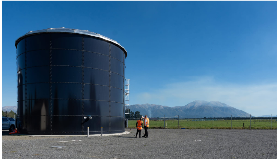
One of the reservoirs at Methven's drinking water treatment plant.
