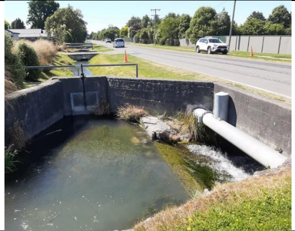
An Ashburton District Council-maintained stock water flow control point at the Creek's northern entry to Methven, flow arriving from the left. (photographed in December 2020). The flow East beside Forest Drive (receding vertically in this photo view) feeds to another stock water branch, and the flow to the right, passing under the road, continues over a concrete weir ledge as Mt.Harding Creek.
