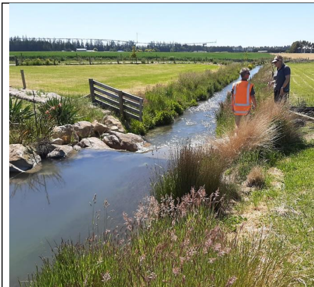
‘Thyme Stream’ landscaping of Creek at new subdivision. Work has included addition of rocks to the stream channel where the resulting flat water behind rock piles acts as a silt trap.
