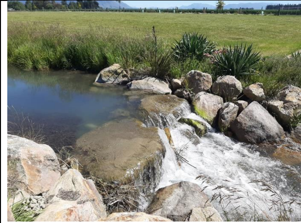
Rocks added to the stream bed at 'Thyme Stream', subdivision on Mt Harding Creek north west of Methven, beside new houses. Silt is settling from the slowed water behind these barriers.
