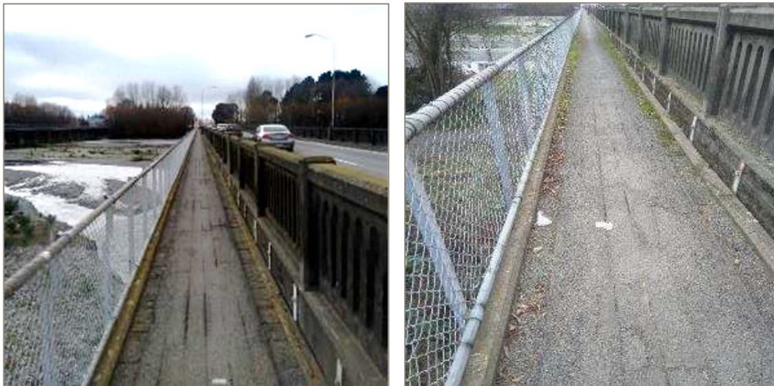
Figure 6-1: Poor quality of existing footpath on the SH1 Bridge
