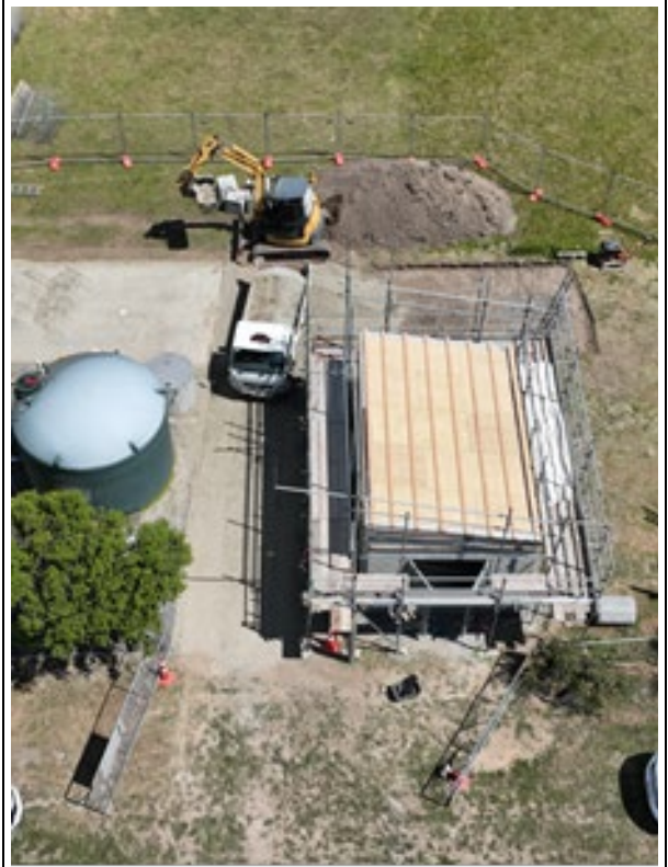
Dromore WTP UV/Filtration Upgrade (ARC Projects Limited)
