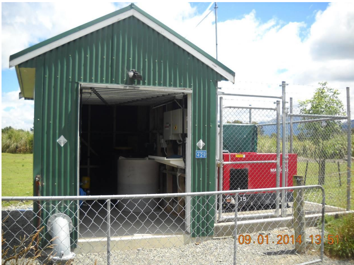
Photograph No 3– Treatment shed with chlorine storage tank and back up generator visible.
