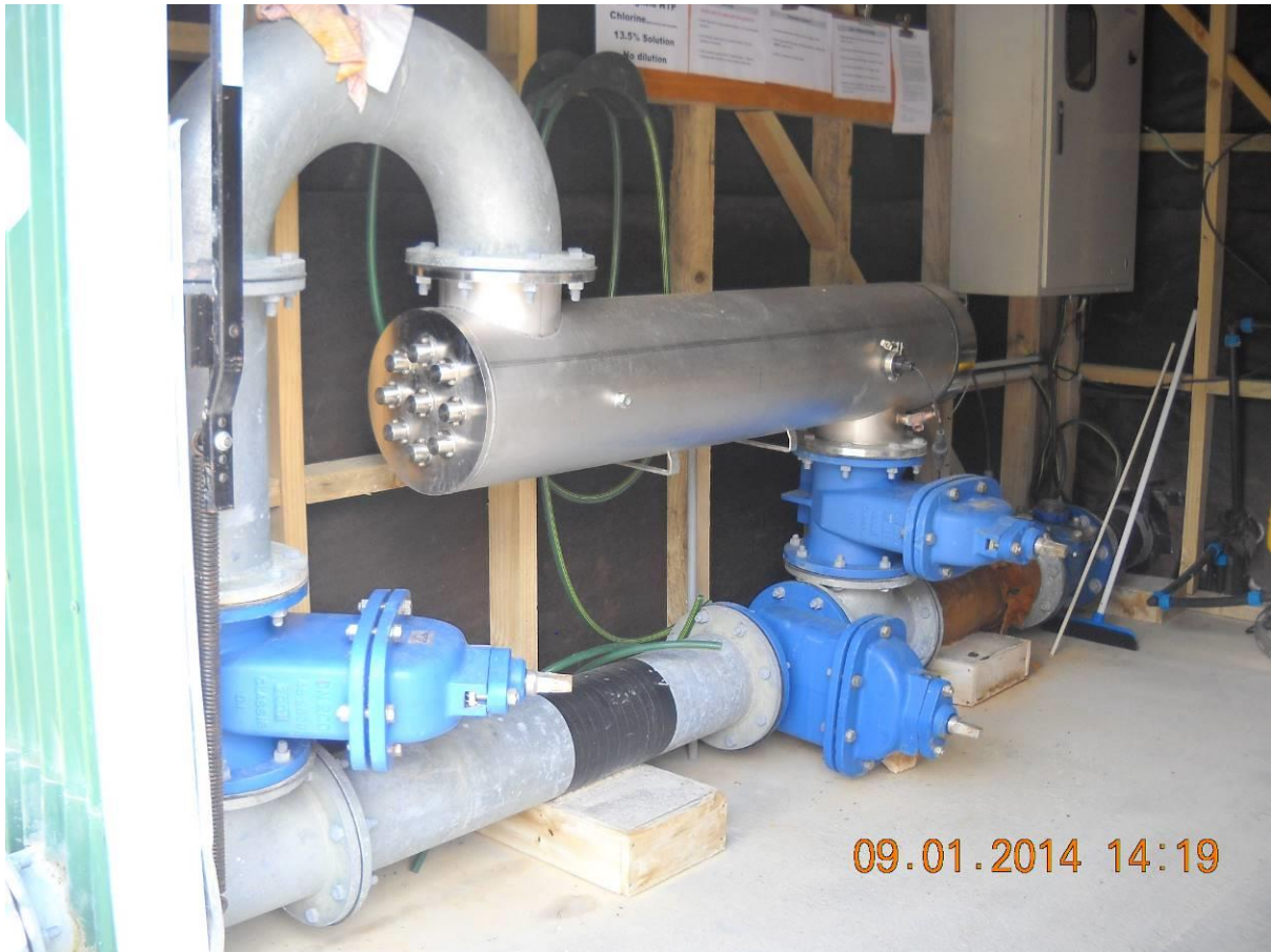
Photograph No 5 – UV unit within treatment plant
