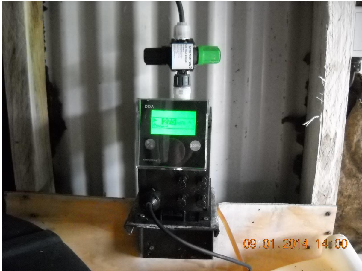
Photograph No 4– Chlorine dosing pump
