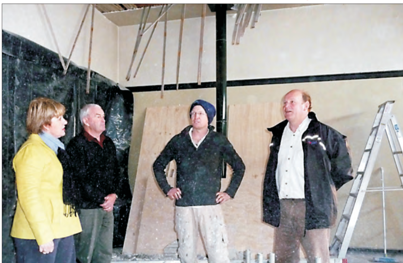
Rangitata MP Jo Goodhew, Methven resident Martin Nordqvist, builder Paul Middleton and Ashburton Mayor Bede O'Malley inspect the damage in Cafe 131 in Methven. The lathe and plaster ceiling is being replaced after earthquake damage, and the popular cafe will be open as soon as possible
